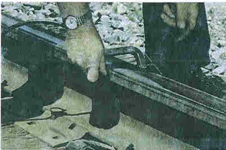
Figure 12-16 Connecting a hardwire shunt on the rail.
