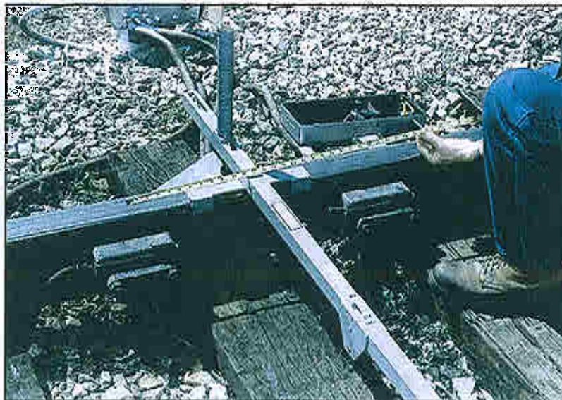
Figure 11-18: Measuring 24 inches between the A and B transducers
